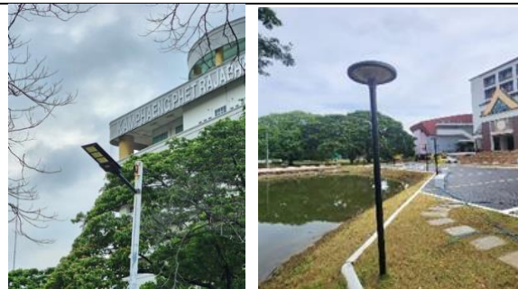
Solar Street lamp
