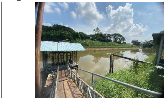
Water intake pipe for treatment process
