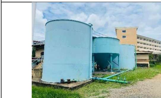
Water treatment facility
